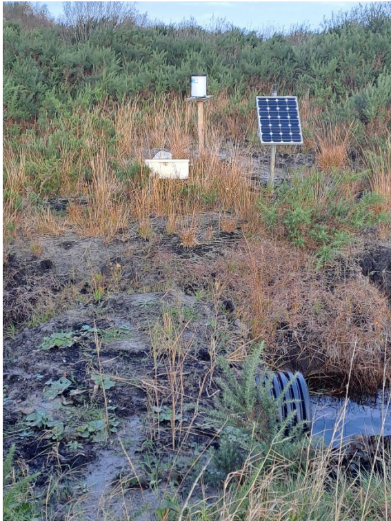
Figure 6.2: Flow Monitoring Velocity probe- Probe is installed in the pipe with the rain gauge, solar panel and container with data logger visible in the background.
