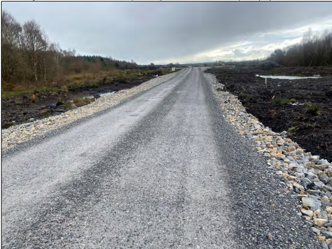
Plate 2-10 Access road associated with the Derrinlough Wind Farm, which is currently under construction since February 2024 classified as Buildings and Artificial Surfaces (BL3)/Spoil and Bare Ground (ED2) recorded throughout the site.
